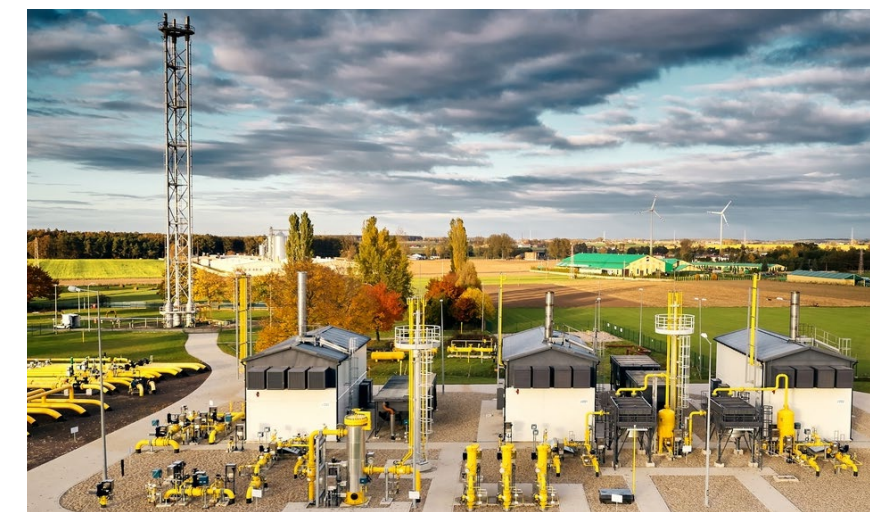
Gas compressor station, Odolanów, Poland.
