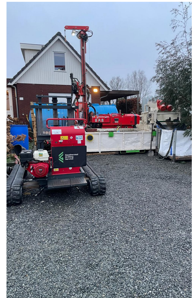
Drilling rig on a driveway for two boreholes with a diameter of 120 mm and 150 m deep. Here, we're using a vibrating screen to collect all the drilling soil in big bags.
