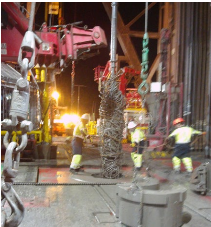
An example of the mess caused by stuck cable.
