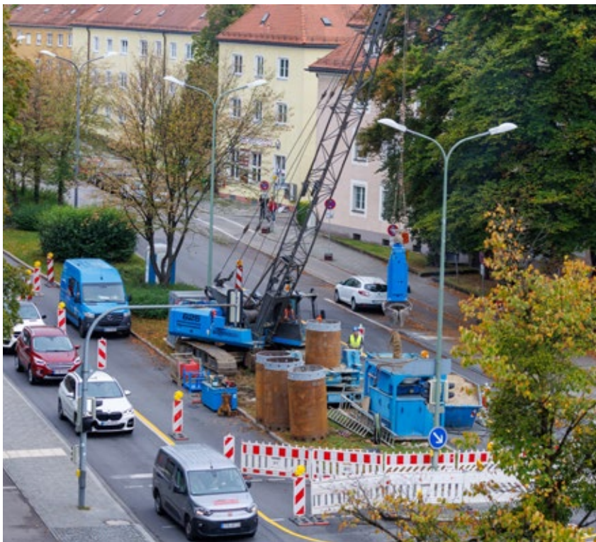
The concrete rings of this shallow geothermal project in the Munich area are stacked on top of each other, after which the sediments are being excavated from the inside. When they reach a certain depth, the horizontal drilling starts, in several directions. These pipes are much smaller.
