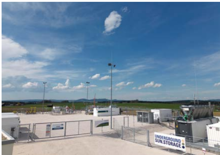
Rubensdorf hydrogen injection facility.
