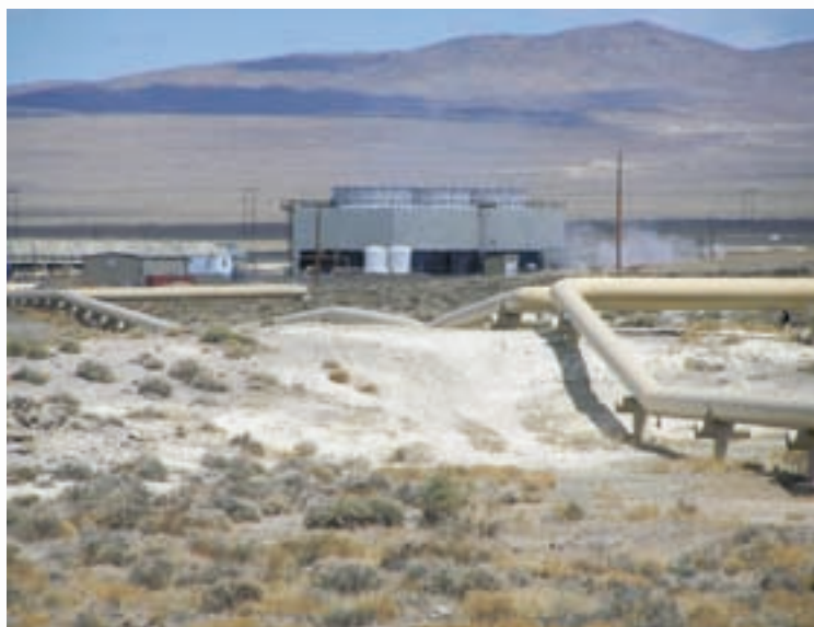
Gathering lines to and from the power plant, both to supply the plant with steam and hot water, and return water back to the injection wells that keep the system charged.
